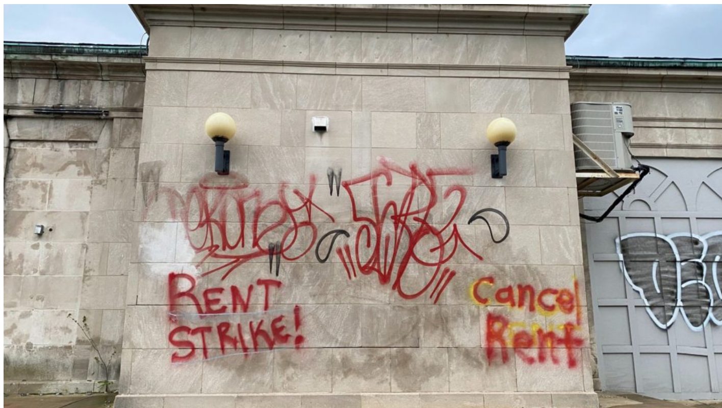
‘Cancel Rent’ graffiti at 23rd and P Street Bridge
